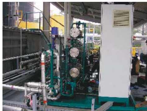
ESSORP -Unit with SPS installed close to the Tankfarm from a Power Plant
