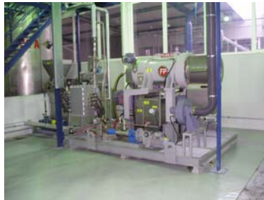
Special designed 3-Phase Decanter for separation of free water / free oil and solids
