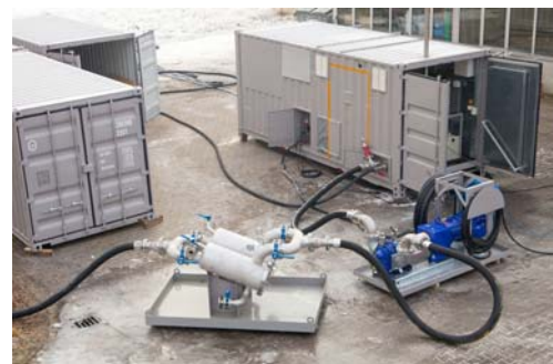
Twin Filter & Suction Pump ready for operation
