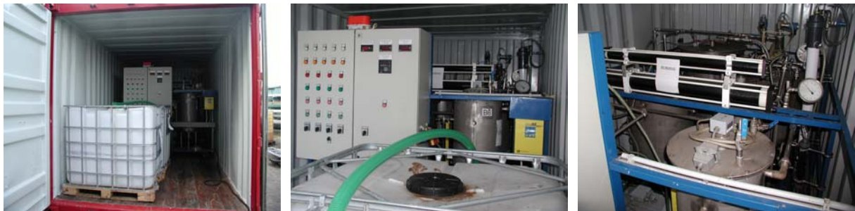
view into the 20 feet container with the installed Membrane-Test Plant
