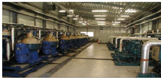
View into the separator room
