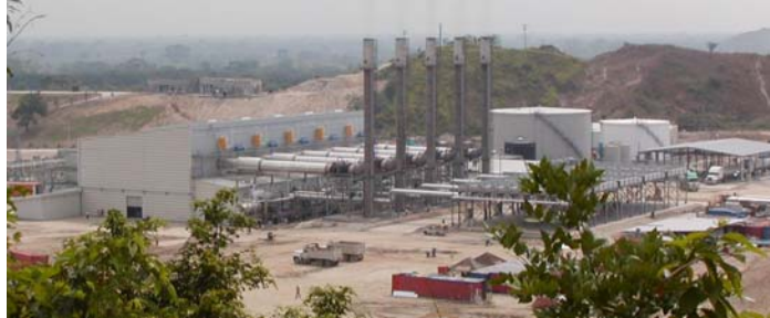
View of the Power Plant at Choloma / Honduras during the first phase of construction with 5 motors for 80 MW installed power
