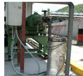
Parts of the ESSORP -demonstration plant
