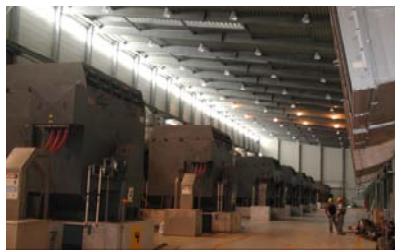
View into the engine room with 13 installed motors
